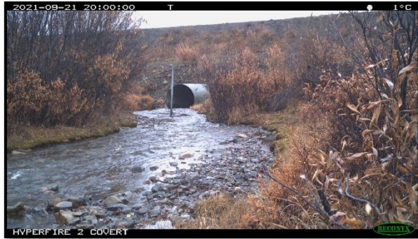
Figure 19. Slavin Creek (km 98.6) timelapse photo of culvert head on September 21, 2021 (Photo provided by McMaster University, Sean Carey’s research team).
