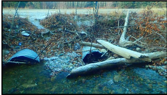
Figure 48. Head of three culverts in the Montague roadhouse rest area in October 2022 (culverts are mostly blocked by debris).
