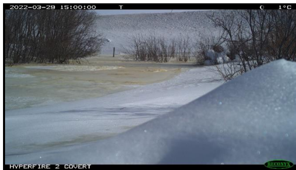
Figure 20. Slavin Creek (km 98.6) timelapse photo of culvert head buried by aufeis on March 29, 2021 (Photo provided by McMaster University, Sean Carey’s research team).
