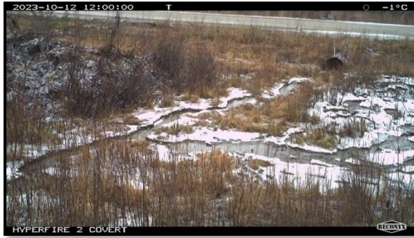
Figure 32. Timelapse photo of Glacier Hill Creek (km 60.1) culvert heads on Oct 12, 2023.
